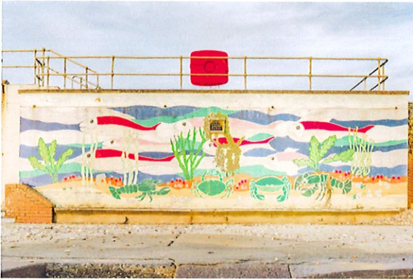
Existing, Verena Sparrow's original mural which has been subject to weather and has been damaged.
